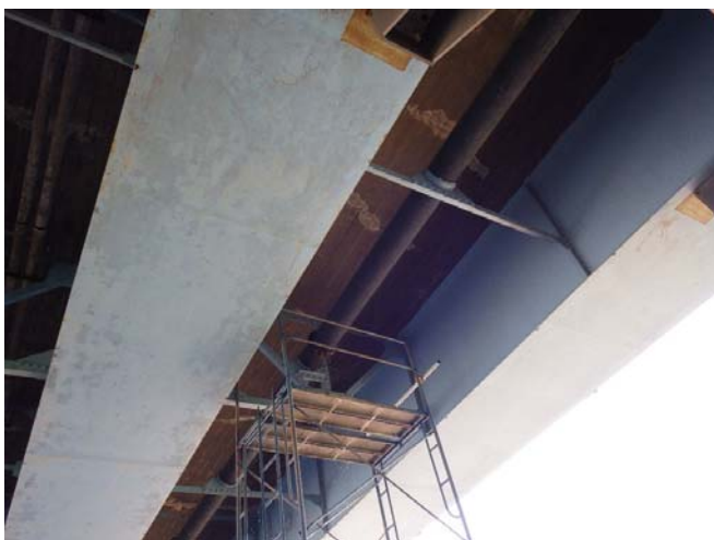
添架管の漏水(1)
