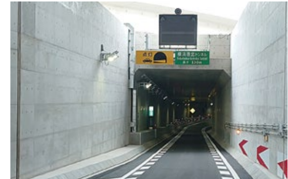
Ramp section box culvert structure at Kohoku Junction, Metropolitan Expressway (Kanagawa Prefecture)
