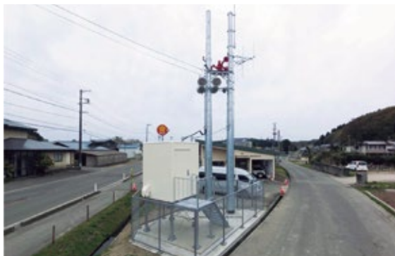
Asahikawa Dam Discharge Warning Station (Akita Prefecture)
