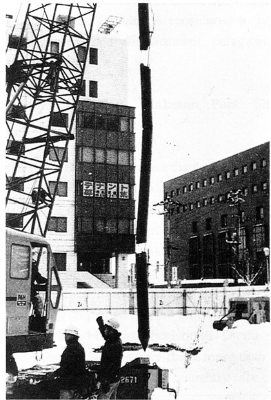
Photo 3-8 Damage to RC pile (Courtesy of Dr. S. Kawamura, et al.)
