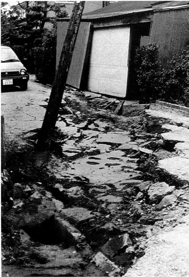
Photo 2-3 Cracks with subsidence on road in Aoba-cho (Courtesy of the Noshiro City Government)
