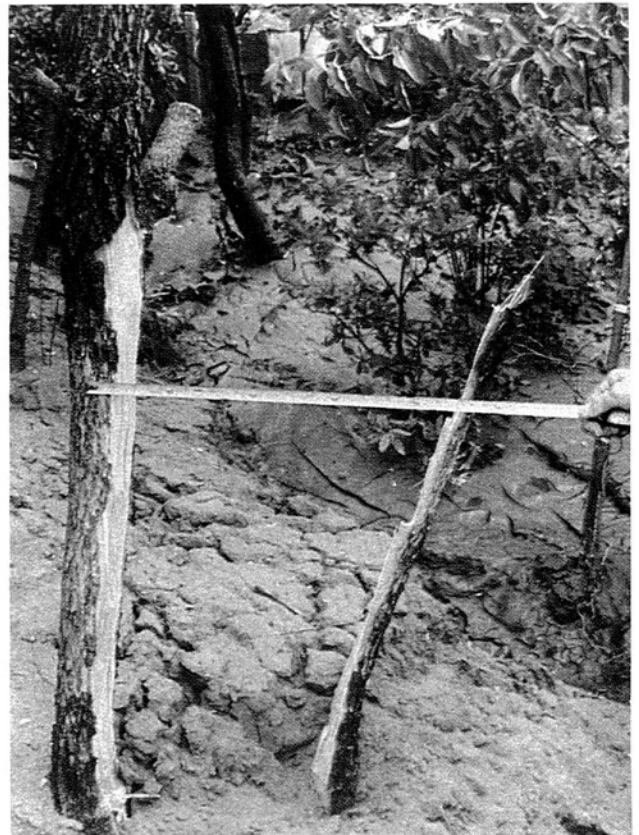
Photo 2-4 A vertically split tree due to liquefaction in Aoba-cho (Courtesy of the Noshiro City Government)
