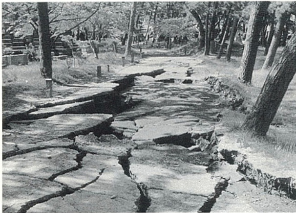
Photo 2-5 Cracks in the road leading to the graveyard in Aoba-cho (Courtesy of the Noshiro City Government)
